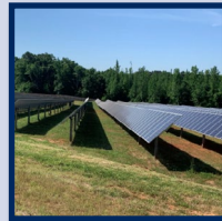
Greene County Solar Facility Hecate Grid Year Complete: 2022 Coxsackie CENTRAL ENERGY/RESILIENCY
